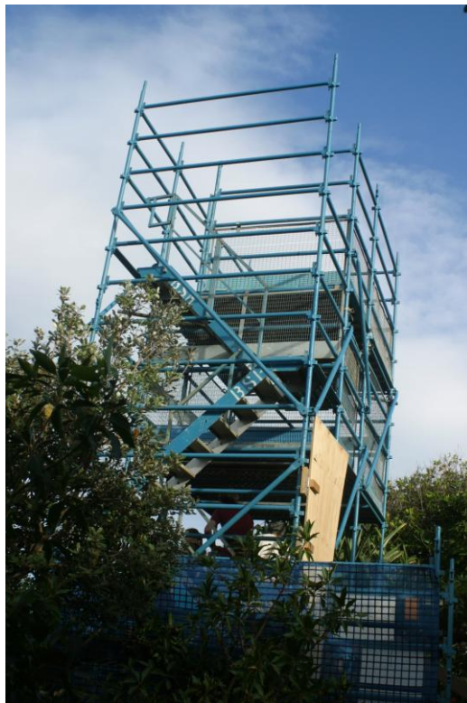
Figure 4. To get around the problems of view, use by rate payers, stability, etc, the Council elected to fund and have built for us a scaffolding tower and platform for our exclusive use above the existing wooden platform. While the initial platform had a floor height of approximately 5m above the ground (pictured here) the tower was much higher than required and the excessive height caused some instability. The top of the tower was therefore dismantled to reduce the height to the floor to about 3m from the ground.
